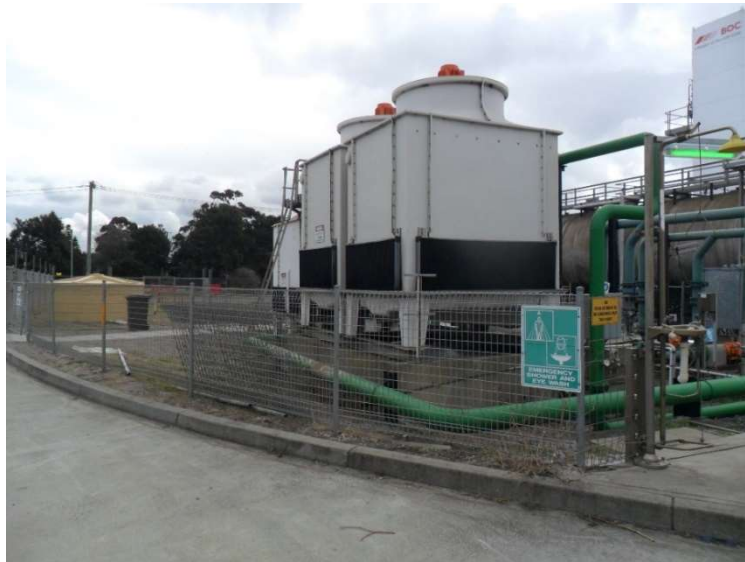
Figure 3-4: BOC Kooragang cooling towers
