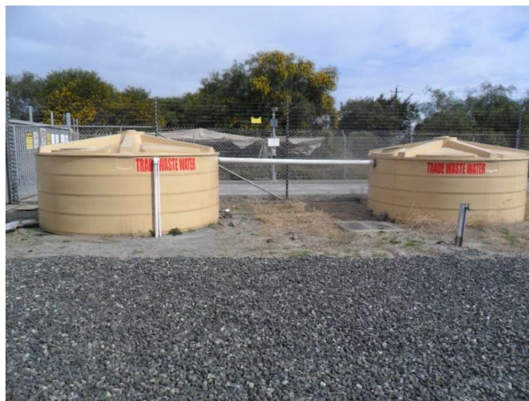
Figure 3-3: Current cooling tower blowdown wastewater storage tanks
