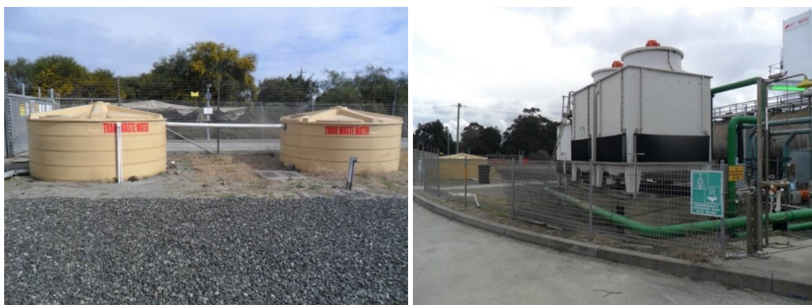
Figure 3.3: Cooling tower blowdown wastewater storage tanks and cooling towers
