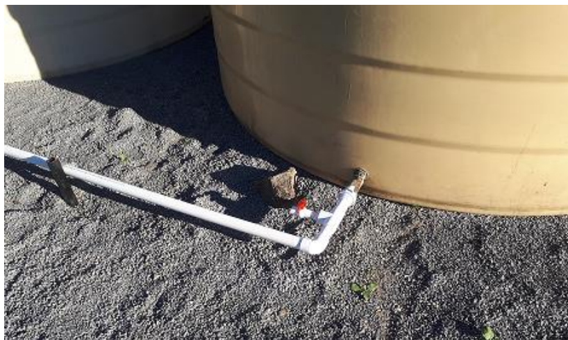
Figure 4-1: Effluent monitoring sample collection point
