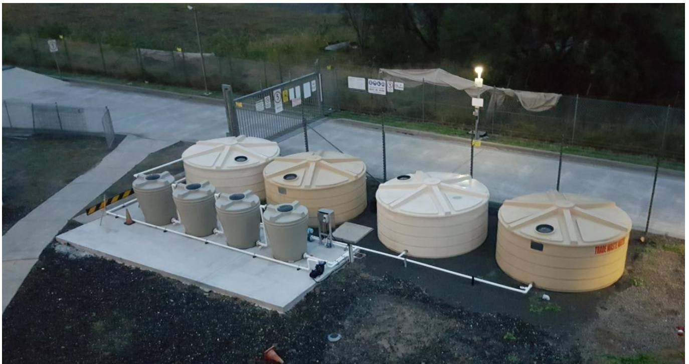
Figure 3-6: Installed pre-treatment system and storage
