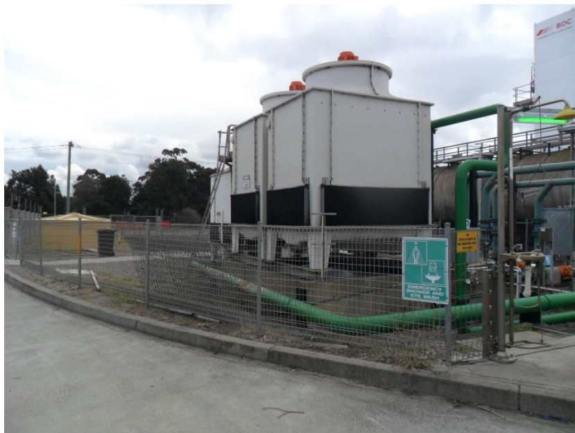
Figure 3-2: BOC Kooragang cooling towers
