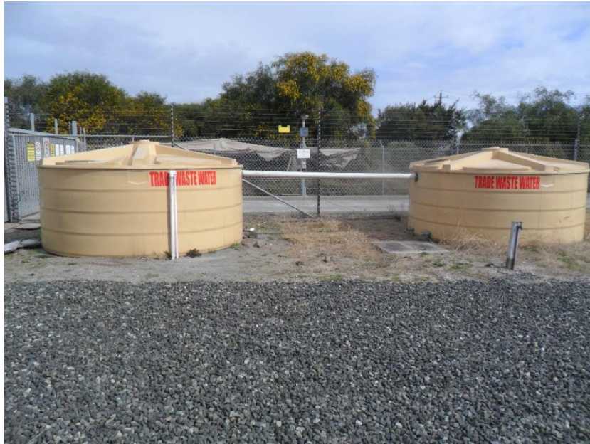
Figure 3-1: Current cooling tower blowdown wastewater storage tanks
